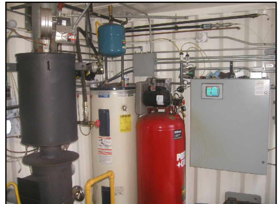
Furnace parts and the PLC touch screen inside the container
